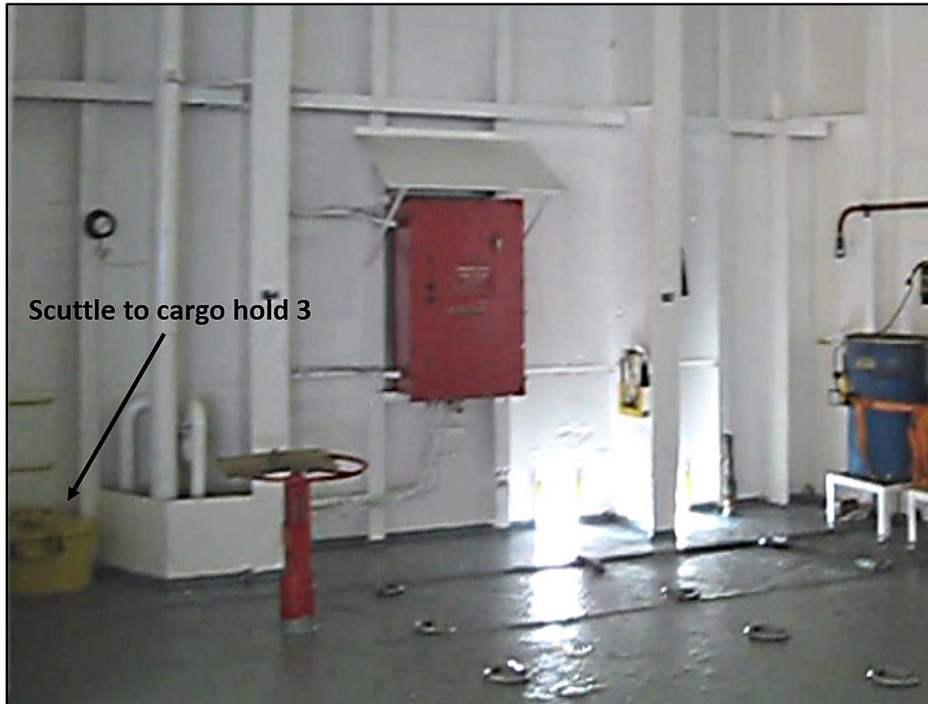
Figure 57. Second deck scuttle to hold 3. (Photo by former El Faro second mate)
